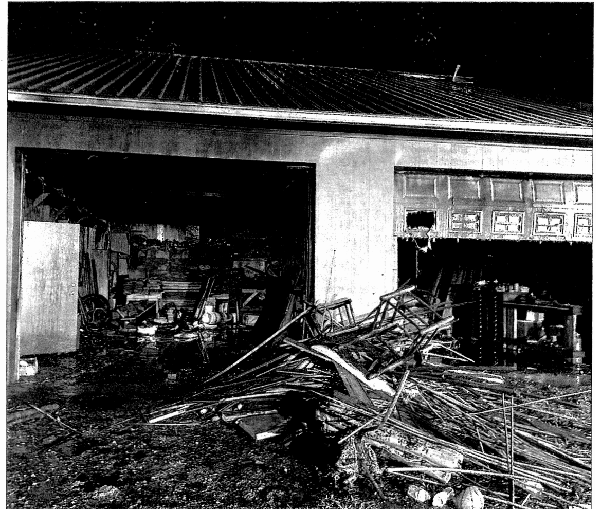
The fire had broken out in the maintenance shop at Black Rock Forest's old headquarters area, on Continental Rd.
